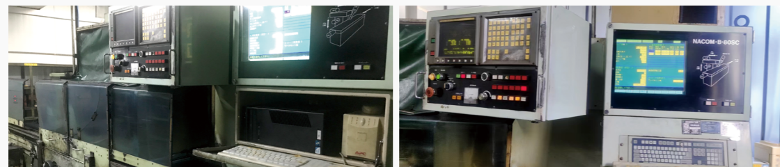
Renewal and Optimization of Old Equipment
