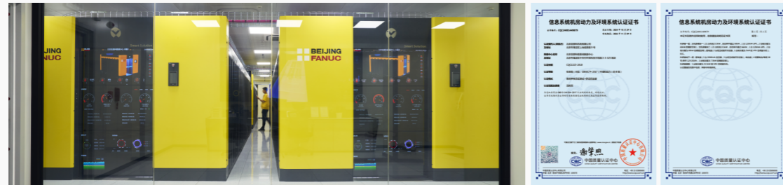
Data Center of BEIJING-FANUC Headquarters Daoxiang Lake Campus
